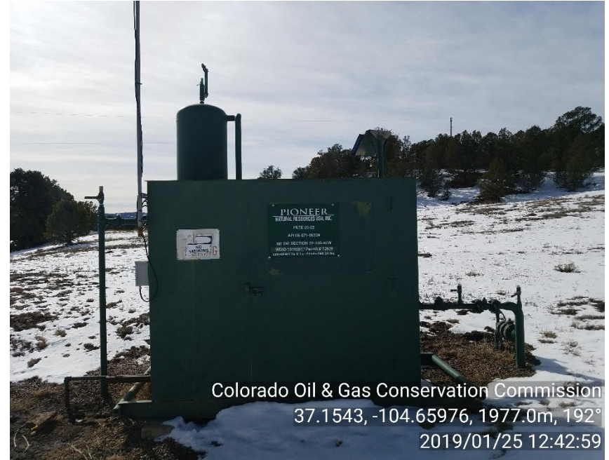
PHOTO 2: WELL SIGN/METER HOUSE
