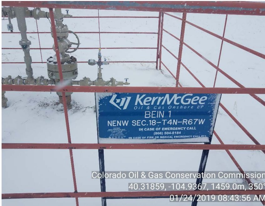
Wellhead sign and emergency contact number
