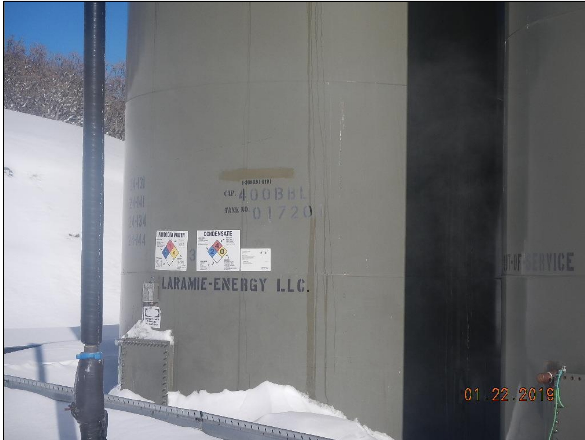
Tank Battery labels
