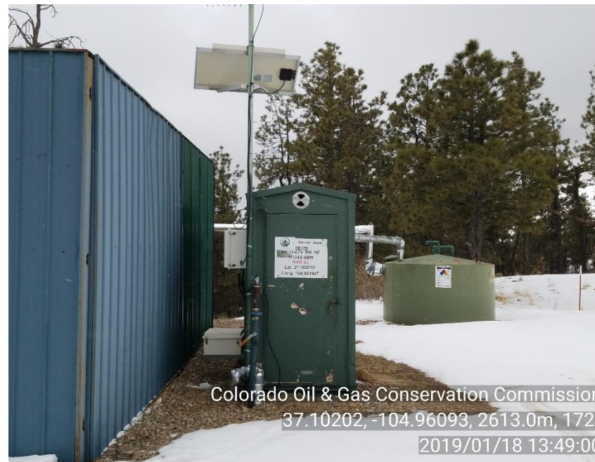
PHOTO 2: WELL SIGN/METER HOUSE
