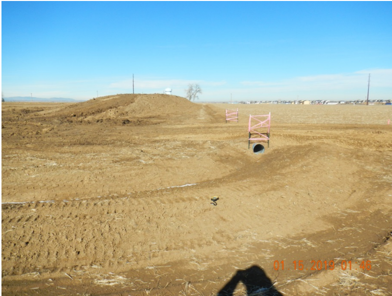
Photo 1. Photo taken from the southeastern perimeter of the location, facing North. Photo illustrates the ditch and berm BMP that has been installed around the perimeter of the location.
