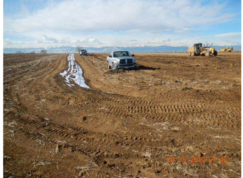
Photo 2. Photo taken from the southeastern perimeter of the location, facing West. Photo illustrates the ditch and berm BMP that has been installed around the perimeter of the location.
