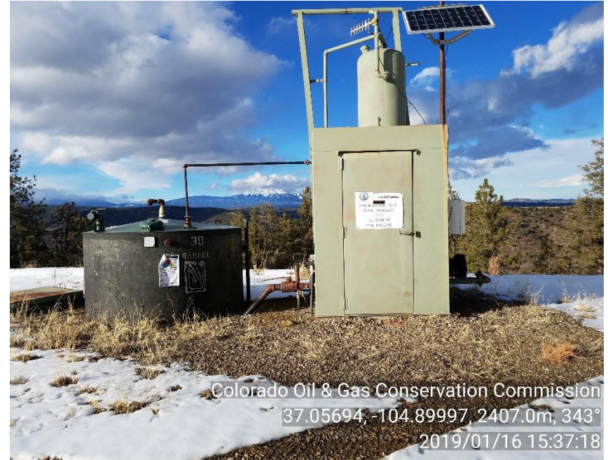
PHOTO 2: WELL SIGN/METER HOUSE
