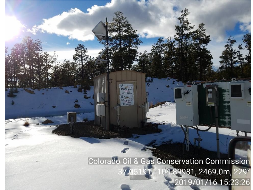
PHOTO 2: WELL SIGN/METER HOUSE
