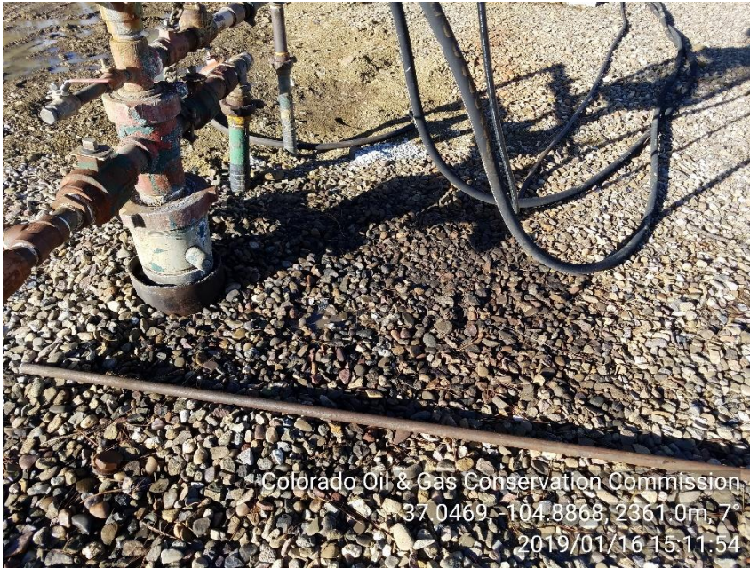
PHOTO 3: STAINED SOIL NEAR WELLHEAD
