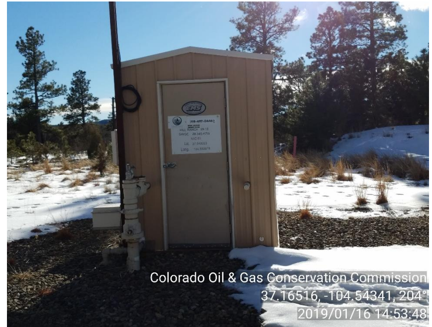
PHOTO 2: WELL SIGN/METER HOUSE
