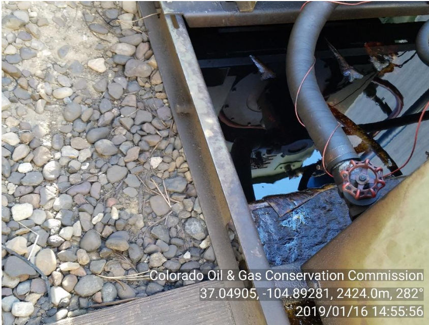
PHOTO 3: STAINED SOIL OUTSIDE ENGINE SKID AT DRAIN PLUG
