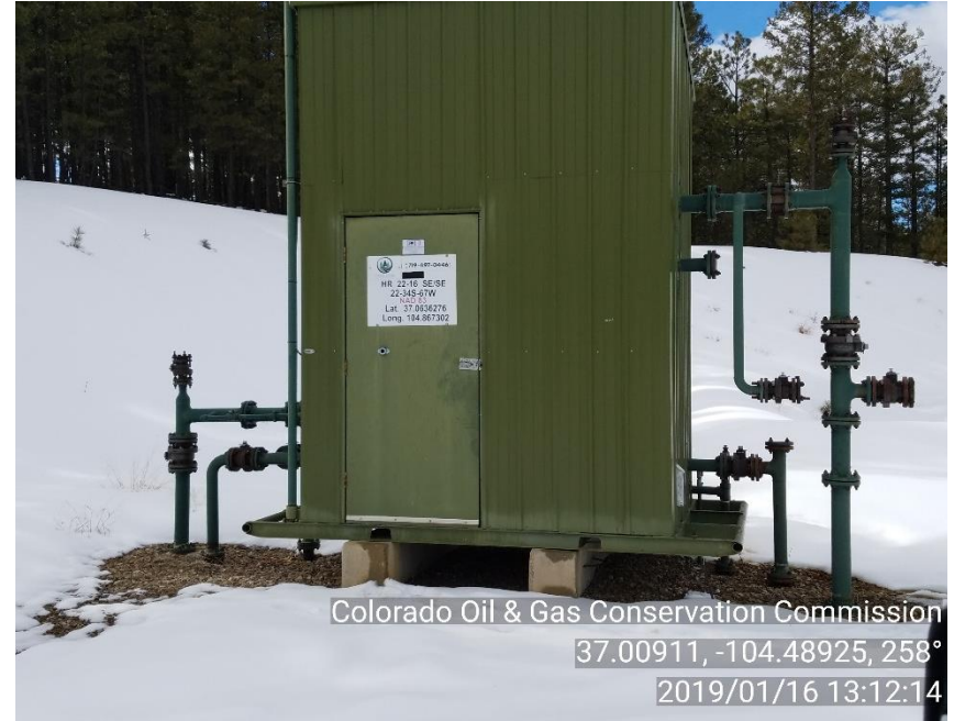
PHOTO 2: WELL SIGN/METER HOUSE
