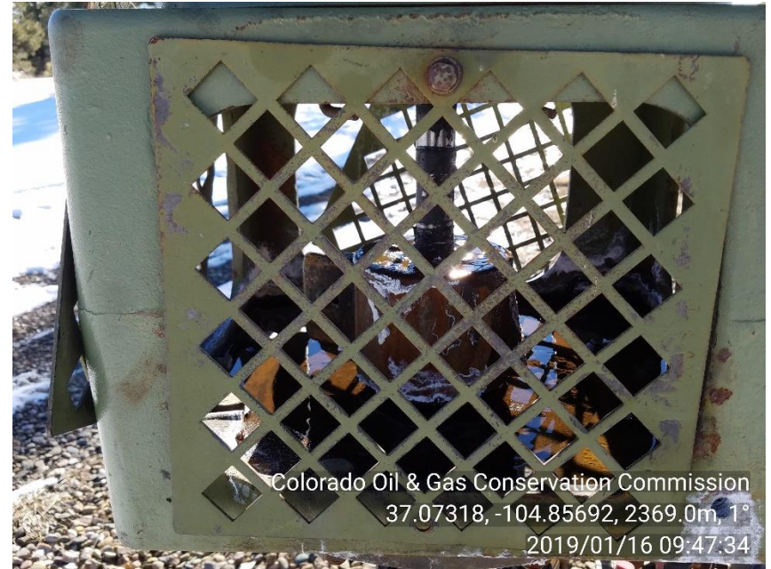
PHOTO 4: FLUID LEAKING FROM ROD PACKING BOX
