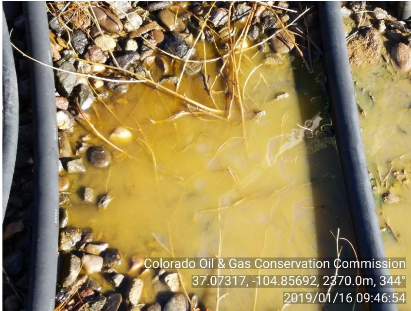
PHOTO 3: OILY APPEARING FLUID FLOATING ON WATER PUDDLE UNDER DRIVEHEAD HYDRAULIC MOTOR
