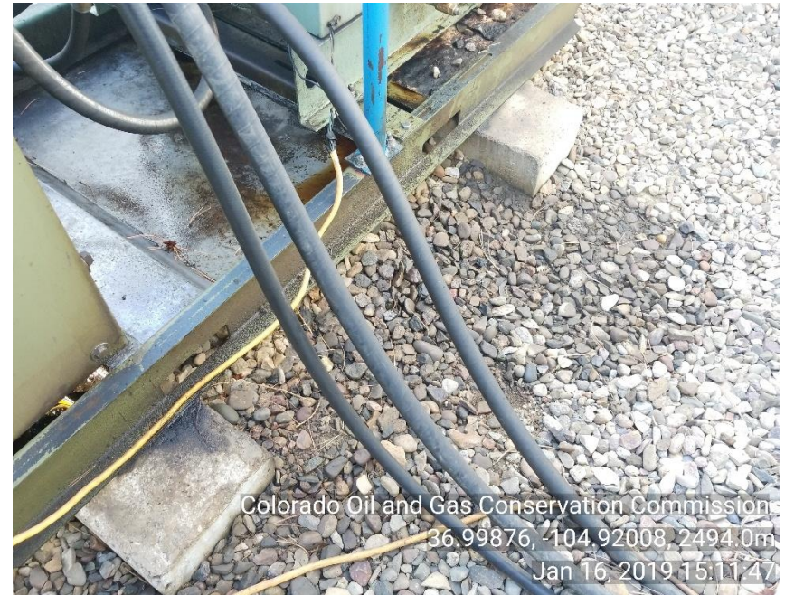
Photo 2 stained soil around motor skid
