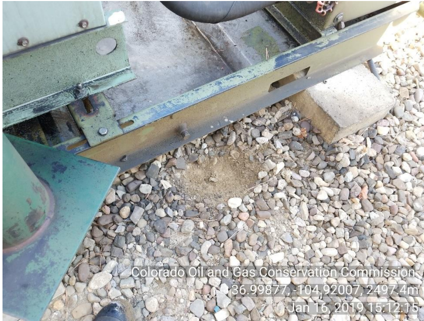
Photo 3 Stained soil around motor skid
