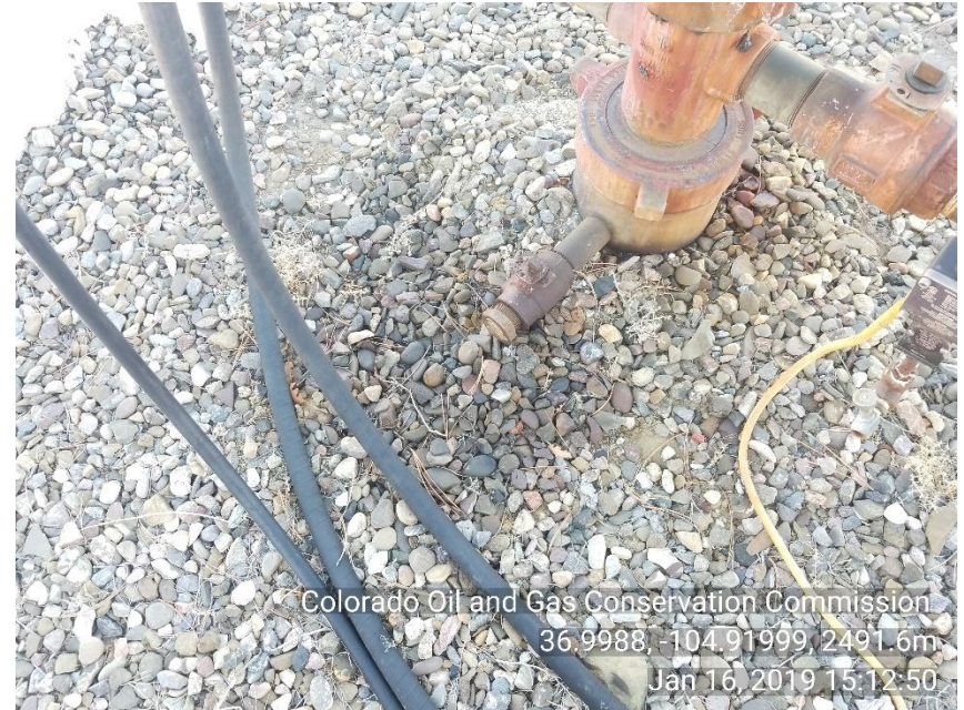
Photo 4 Stained soil around WH under HYD fittings
