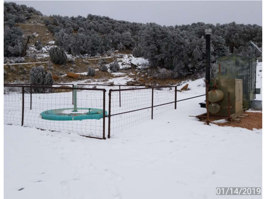
Photo 2. Tank battery, separator, and gas meter building.
