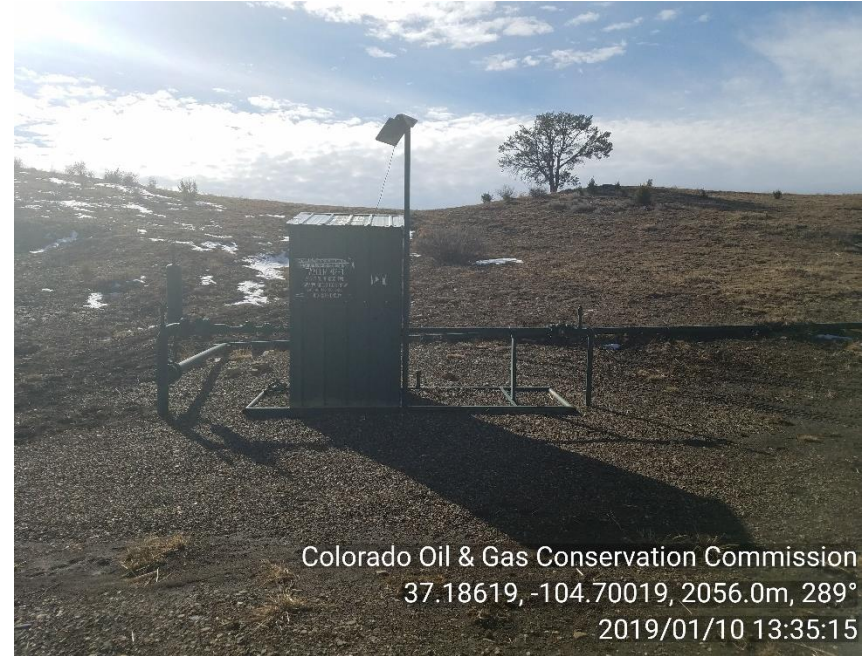
PHOTO 2: WELL SIGN/METER HOUSE
