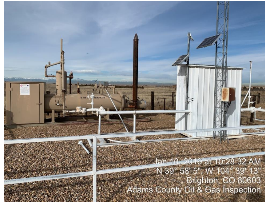
Photo#2 Separator/Gas Meter/Automation RTU
