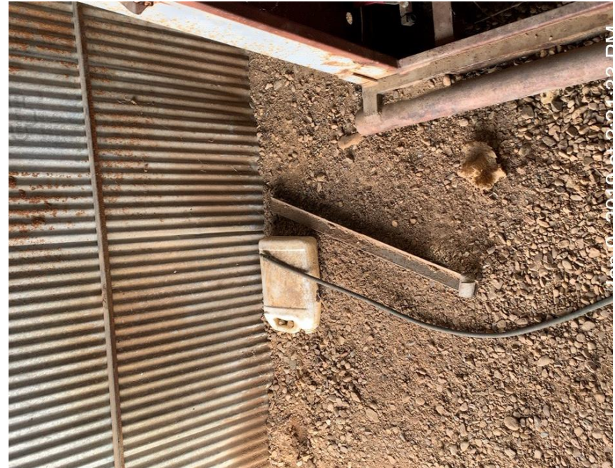
Photo#12 Corrective Action/Trash
