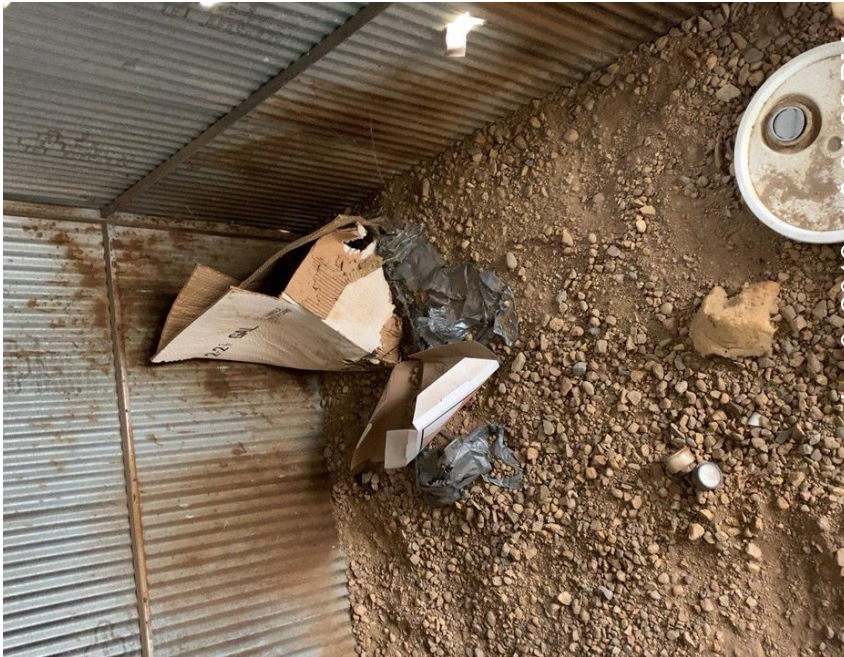
Photo#11 Corrective Action/Trash
