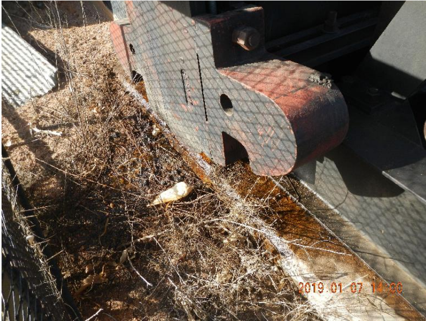
Photo 5: Impacted soil off L side of pump jack.
