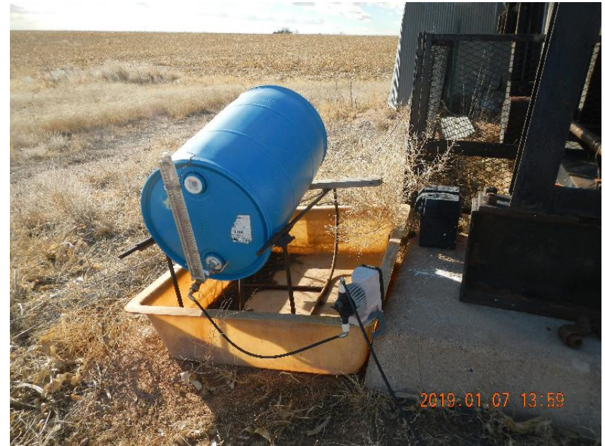
Photo 4: Chemical tank on spill prevention. Chemical pump and battery visible.
