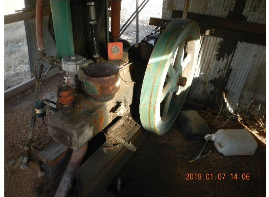
Photo 8: Natural gas prime mover.
