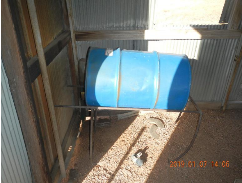
Photo 7: Partial 55 gallon drum of lube oil with no spill prevention.
