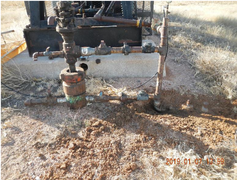
Photo 3: Wellhead tree with exposed valve on R side of tree.
