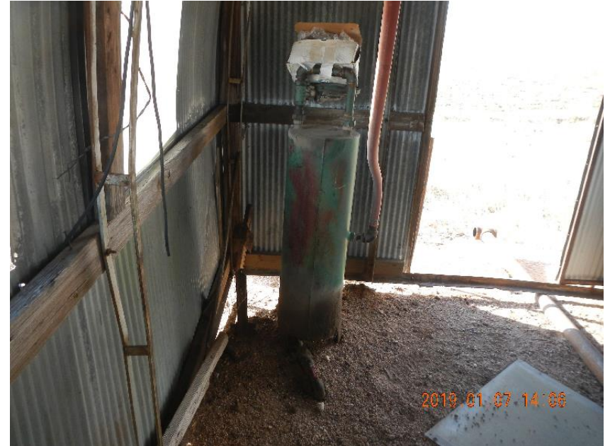
Photo 6: Supply gas knock out with 1" supply gas line coming in at base of knock out.
