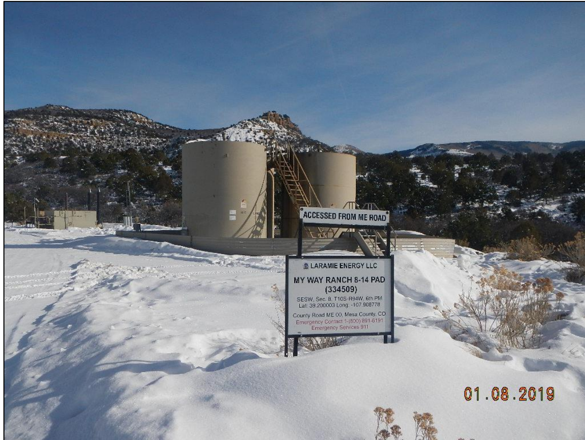
Photo of tank battery sign at entrance of location
