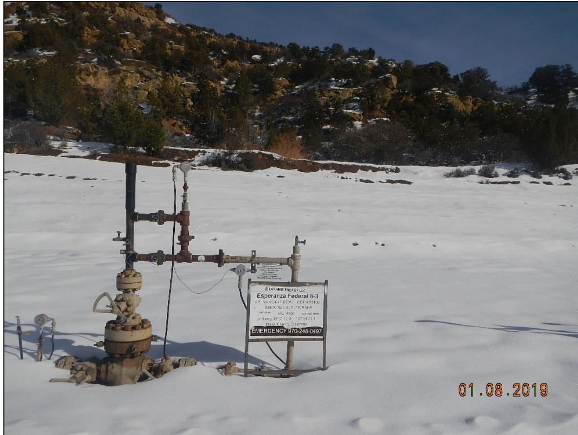
Well head signs in place
