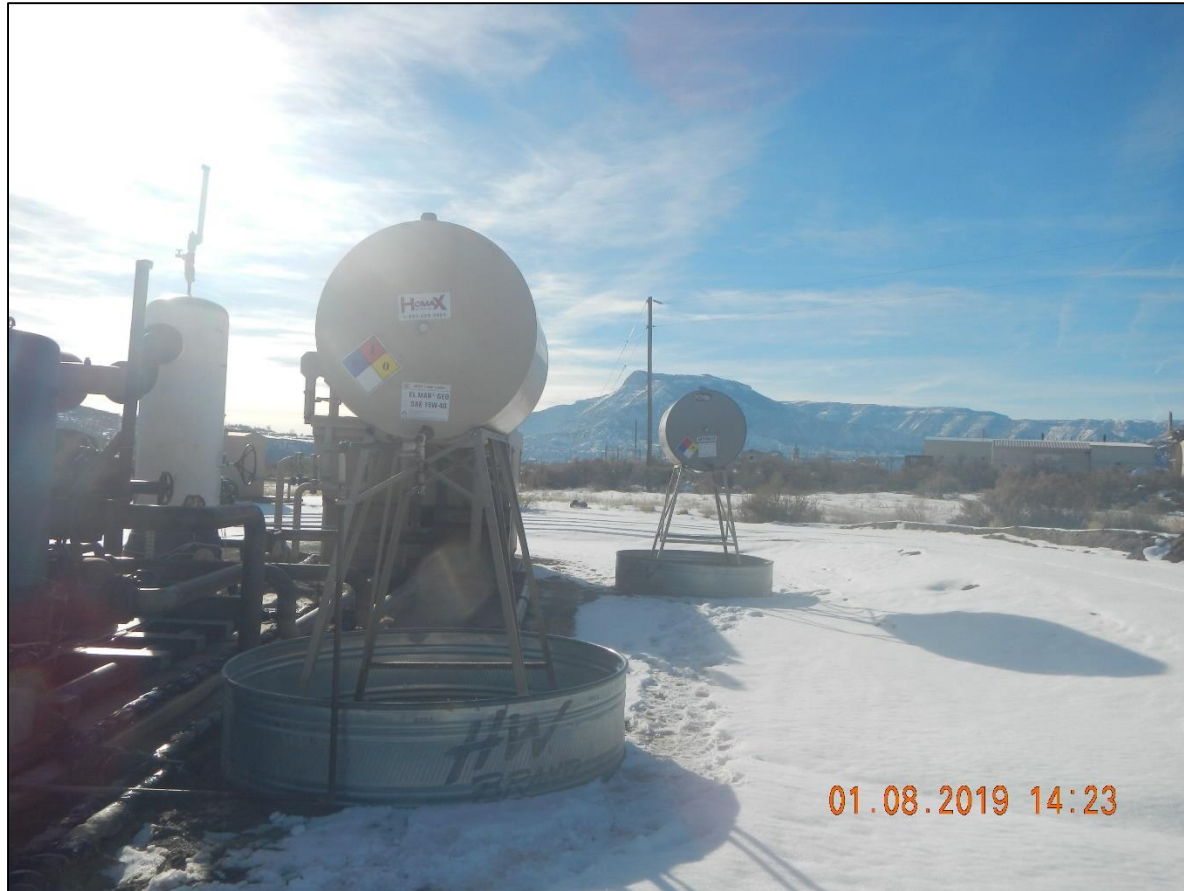
Tank NFPA labels have been fixed.
