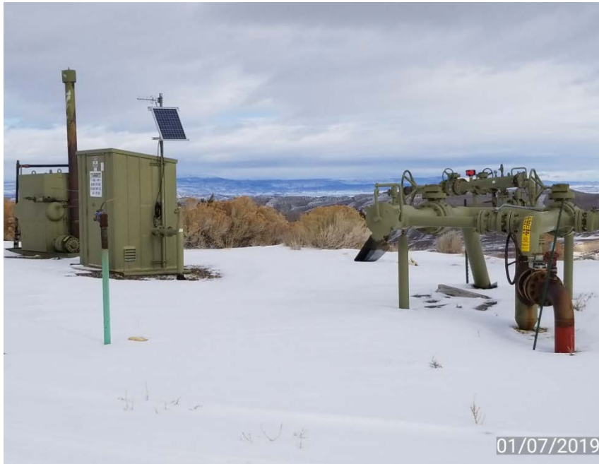
Photo 3. Separator and gas meter building.
