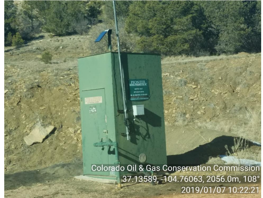
PHOTO 2: WELL SIGN/METER HOUSE
