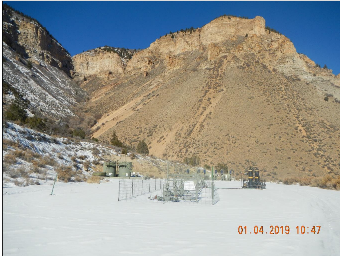
Location photo. Vertical separators at wells.
