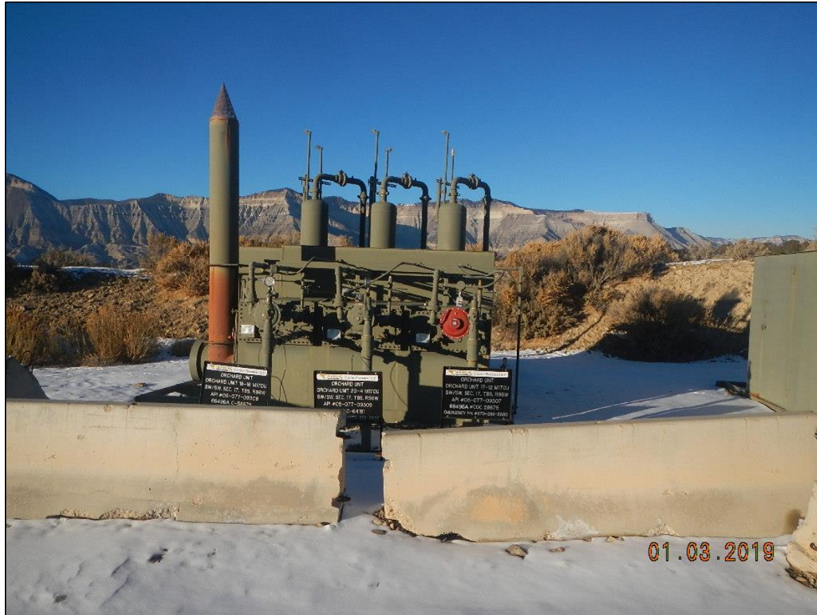
photo of tank battery sign at separators
