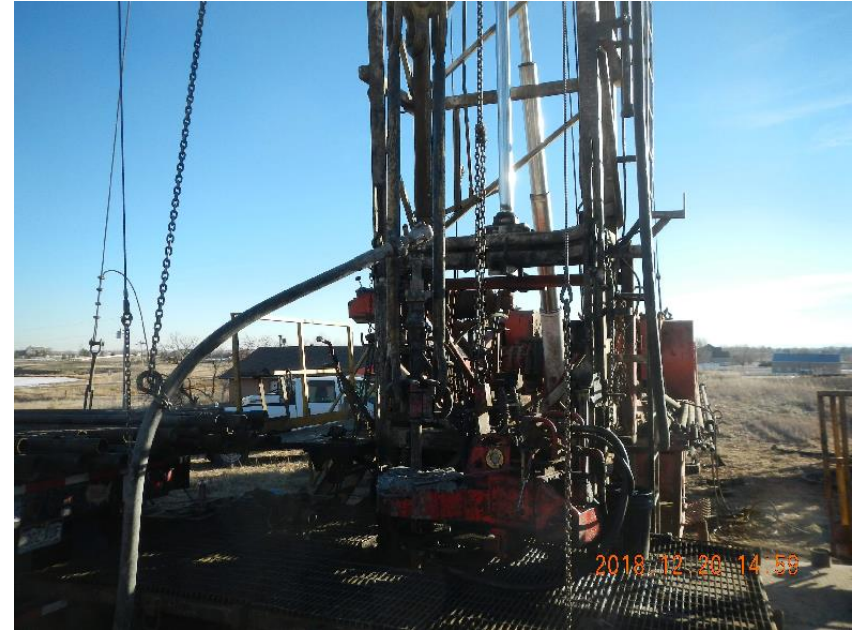
Photo 2: Rigged up to tubing to pump cement down hole for balance plug.
