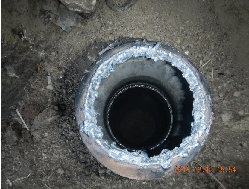
Photo 7: View into well bore after the casing has been cut down to install the 4" swedge.
