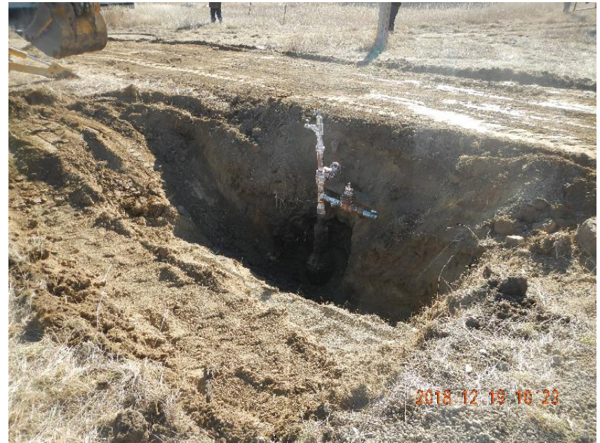
Photo 4: Overview of area around wellhead with S side leveled and compacted for rig balance beam.
