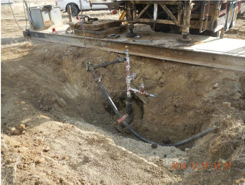
Photo 5: Wellhead plumbed into the transfer pump with the rig balance beam and rig in the background.
