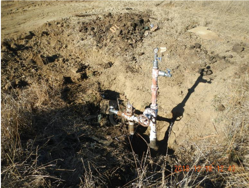
Photo 5: Wellhead with 1" flowline disconnected and bull plug and needle valve installed. Bull plug with needle valve and pressure gauge installed (top).
