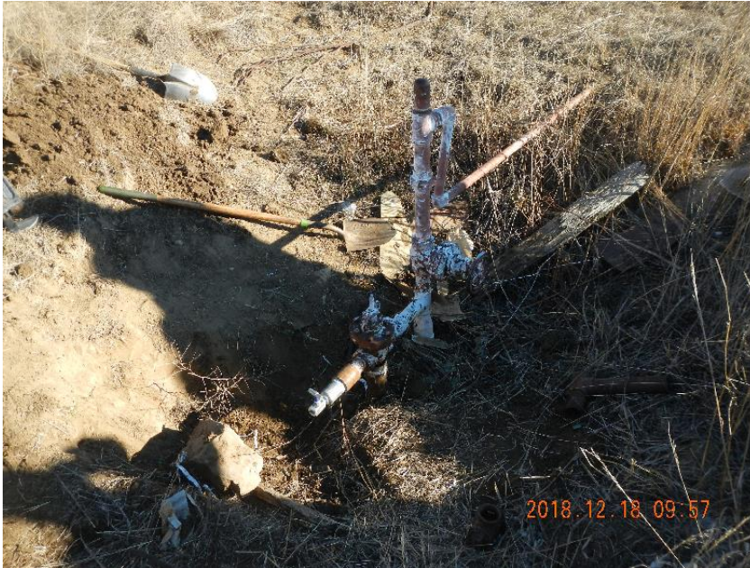
Photo 1: Wellhead with W 2" flowline disconnected and bull plug and needle valve installed.
