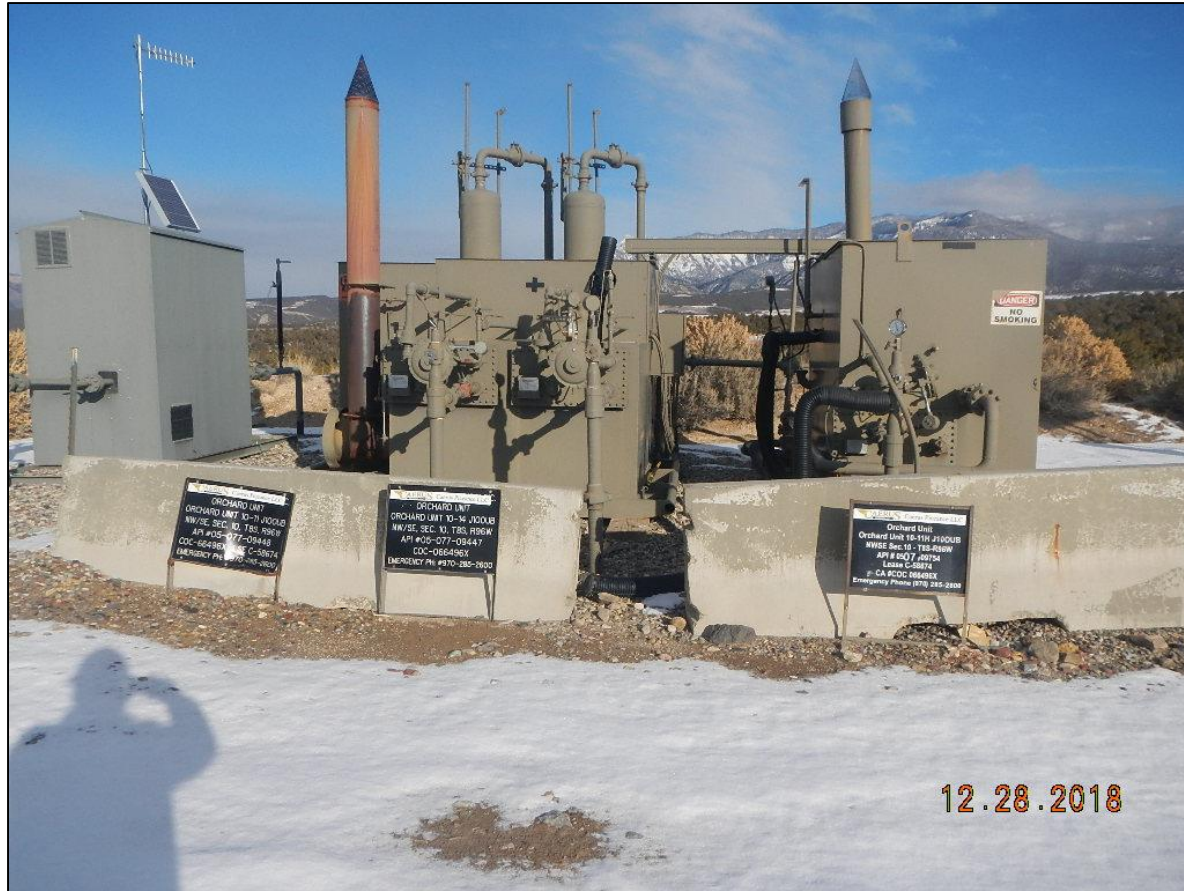
Photo of tank battery sign at Separator
