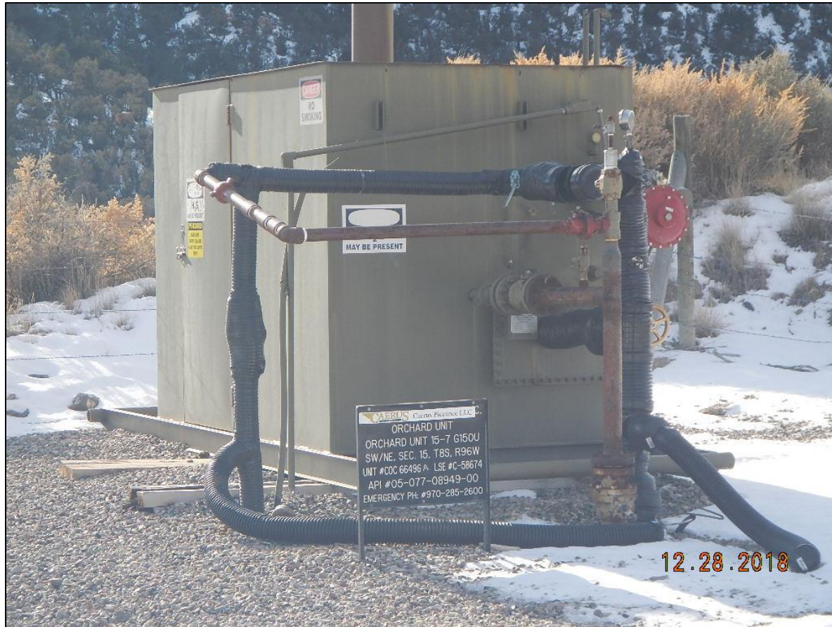
Photo of tank battery sign at Separator
