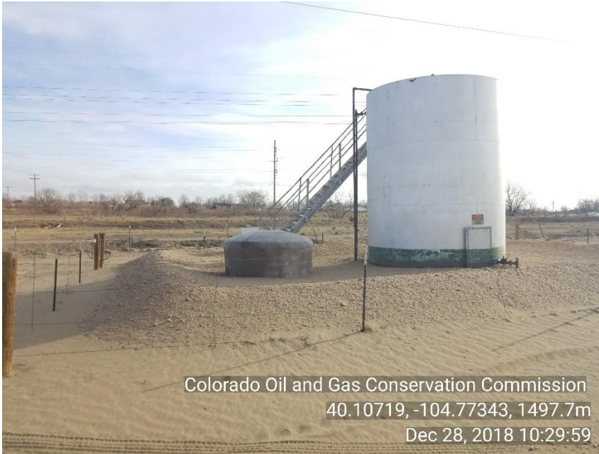
Photo 3 Tanks not painted next to county road
