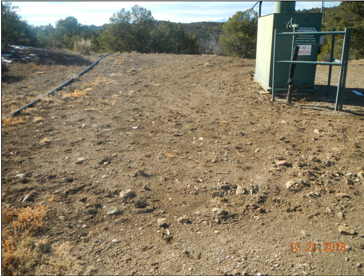
Photo 2. The west side of the location appears to have been disturbed and does not have adequate vegetation cover.
