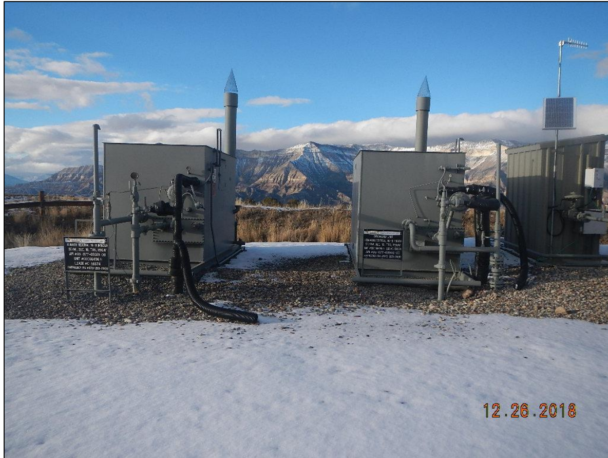
Photo of tank battery at separators
