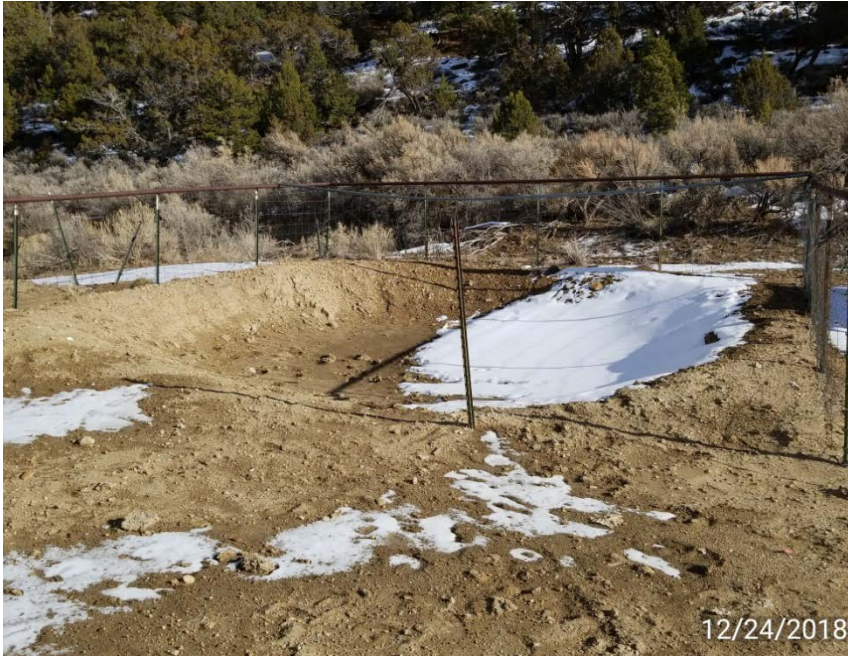
Photo 3. Pit missing fence on one side.
