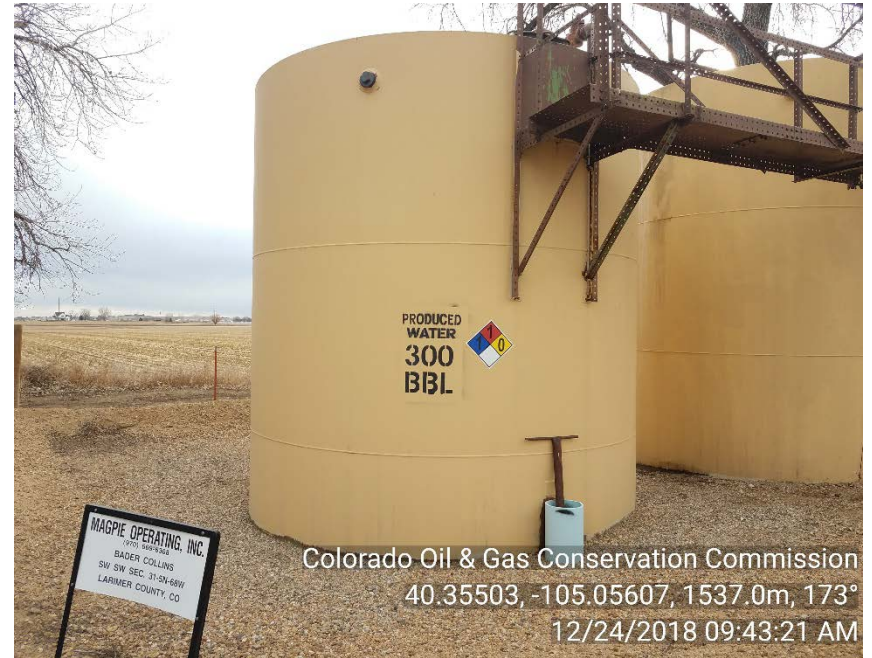
Produced water tank placards on 12/24/18
