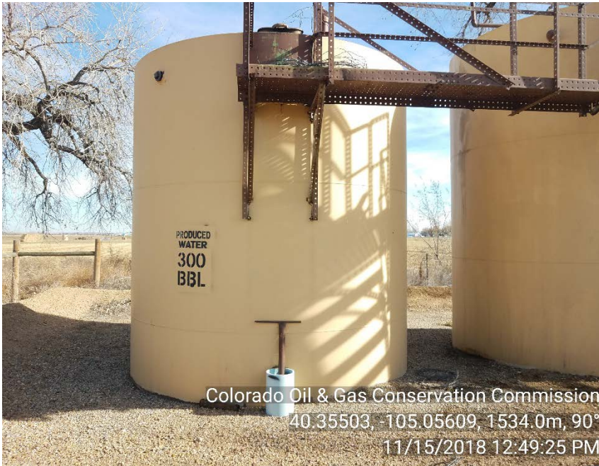
Produced water tank placards on 11/15/18
