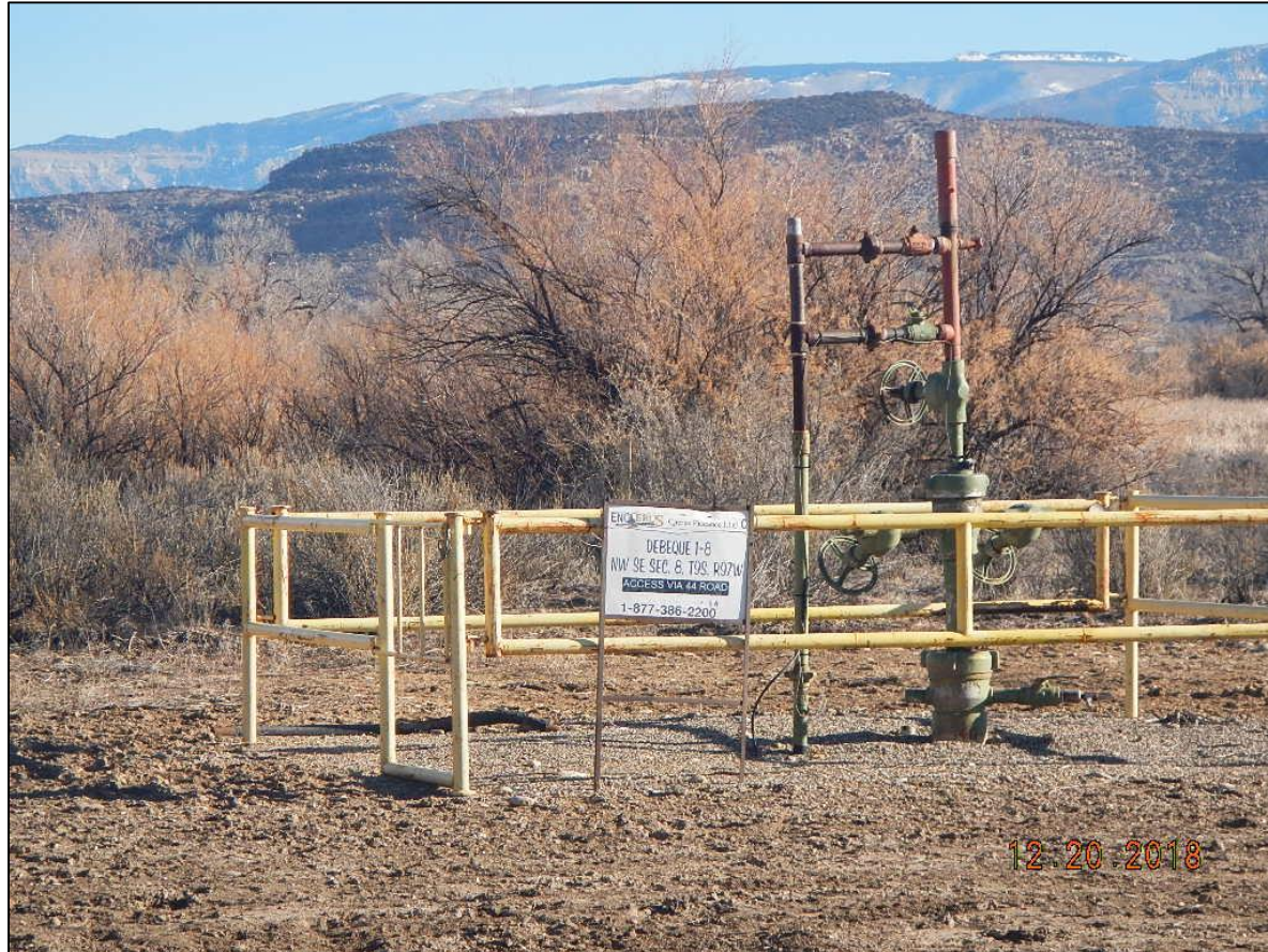
Tank battery sign at wellhead Phone # also listed on tank sign
