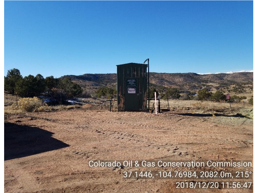
PHOTO 2: WELL SIGN/METER HOUSE
