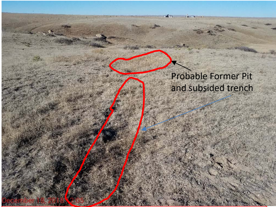
Photo 1 – Looking west toward subsidence along probably pipe toward former pit
