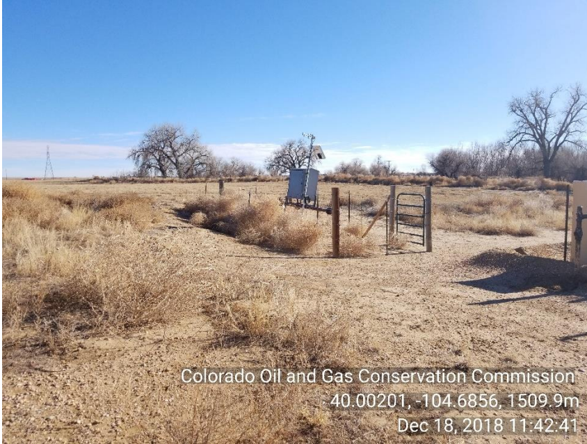
Photo 7 Weeds meter run
