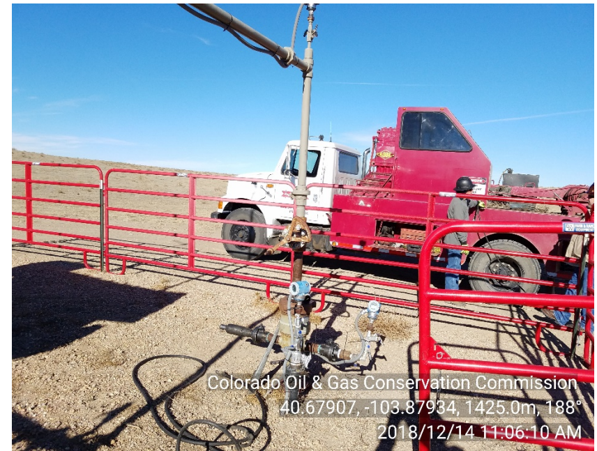
Photo #2 Lilli Unit 8-8 Wellhead – UIC-MIT
