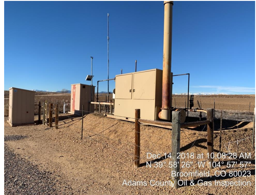
Photo#2 Separator and Gas Meter
