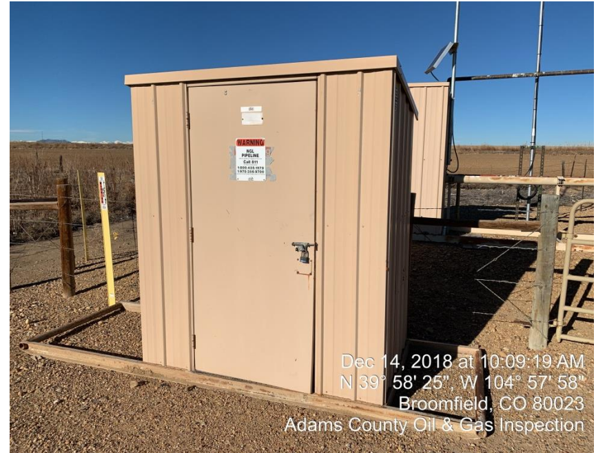
Photo#4 Corrective Action Unused Equipment
