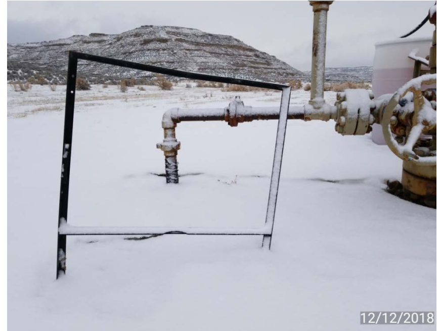
Photo 4. Well head sign missing.
