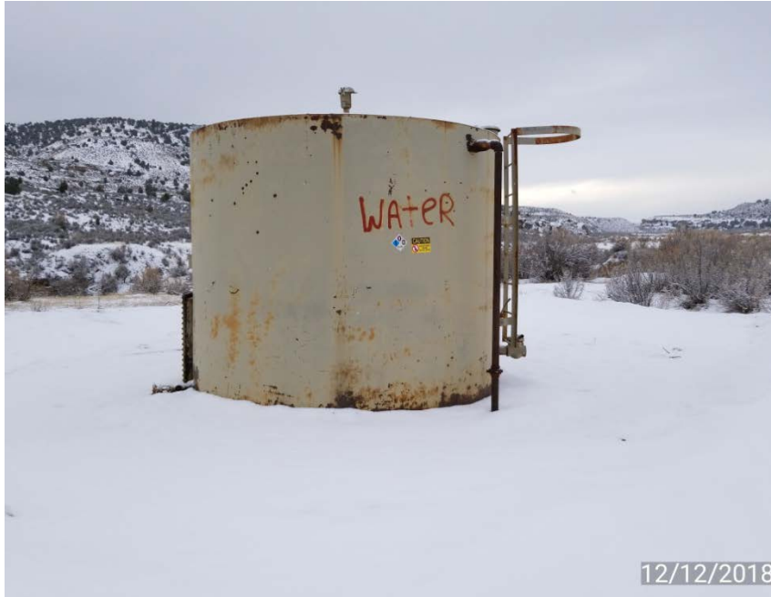
Photo 3. Signage missing capacity of 112 bbl.
