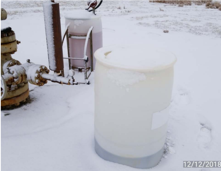
Photo 5. Containers missing label.
