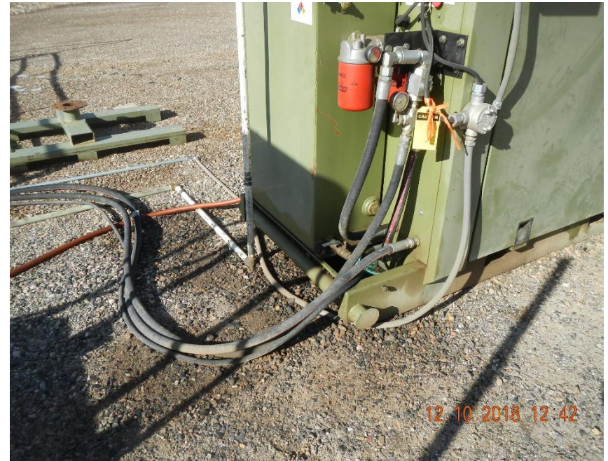
Lube oil leak at Oil Lift equipment.
