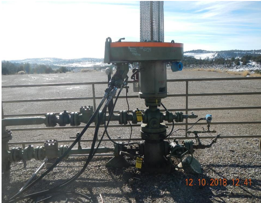
Burkett A #2 well head is tagged out for Spill/Release Point ID #459307.
