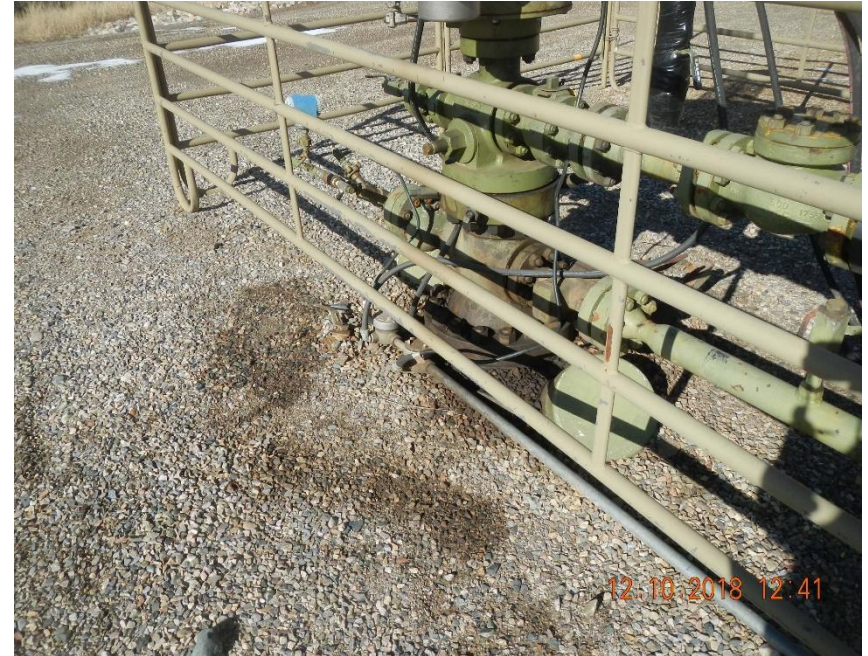
Stained gravel near well head.
