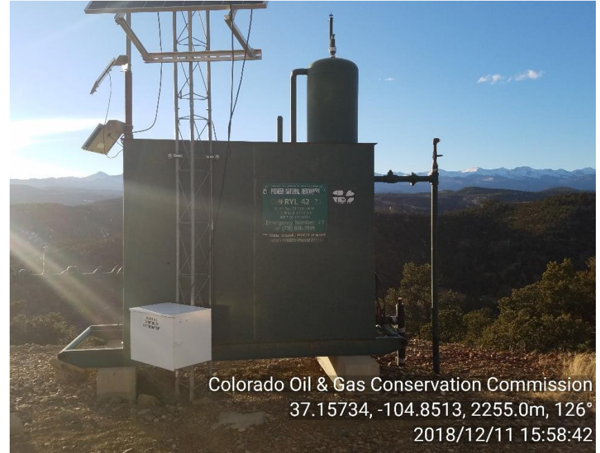
PHOTO 2: WELL SIGN/METER HOUSE
