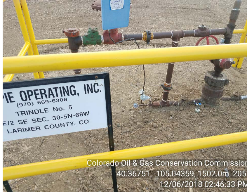
Wellhead and Bradenhead valve
