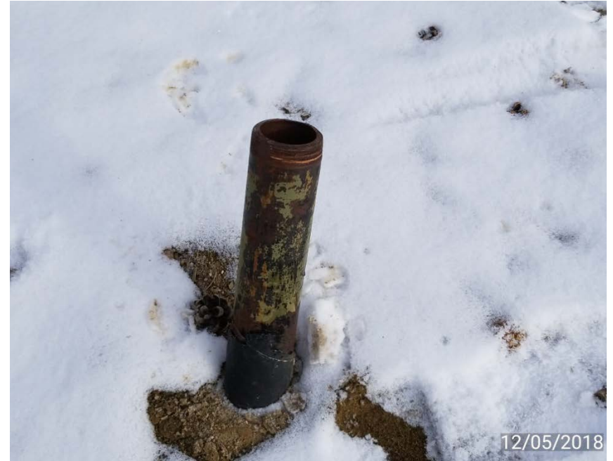
Photo 2. Riser not capped or LOTO.
