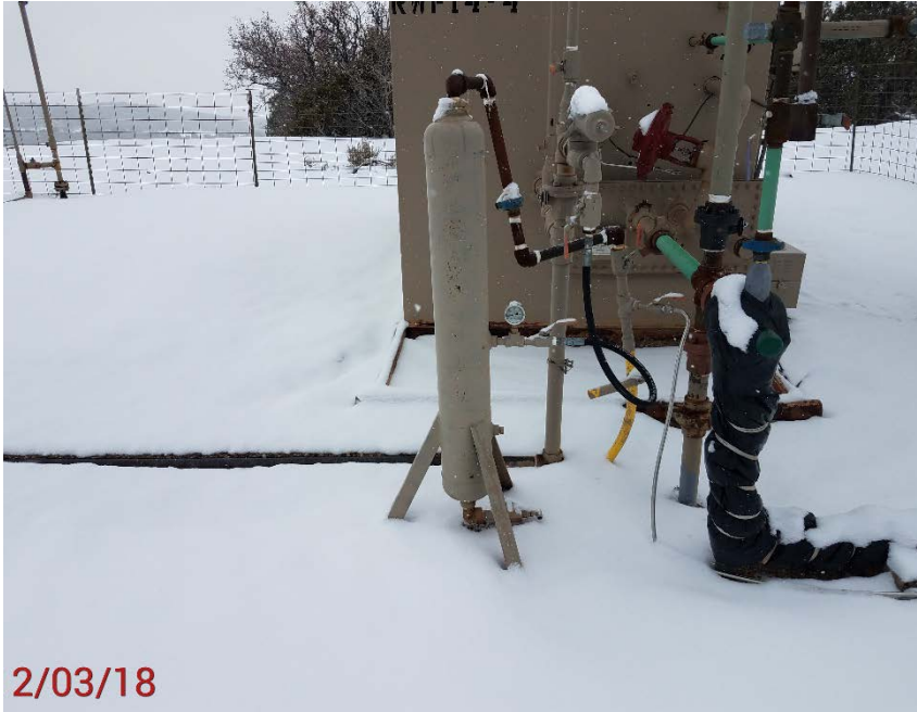
Location Photo #3, Domestic tap
