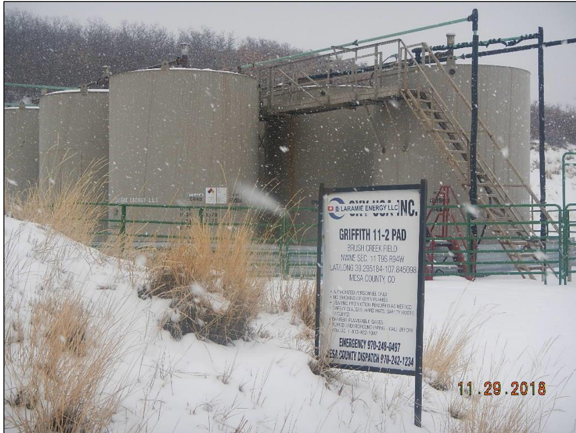
Tank battery sign at entrance of location
