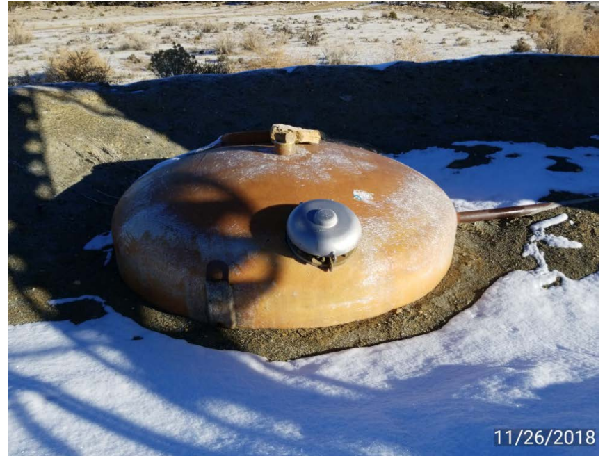
Photo 2. Tank without labeling.
