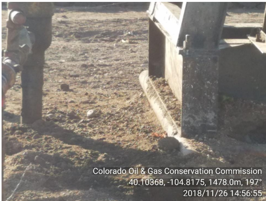
PHOTO 3: STAINED SOIL AROUND WELLHEAD
