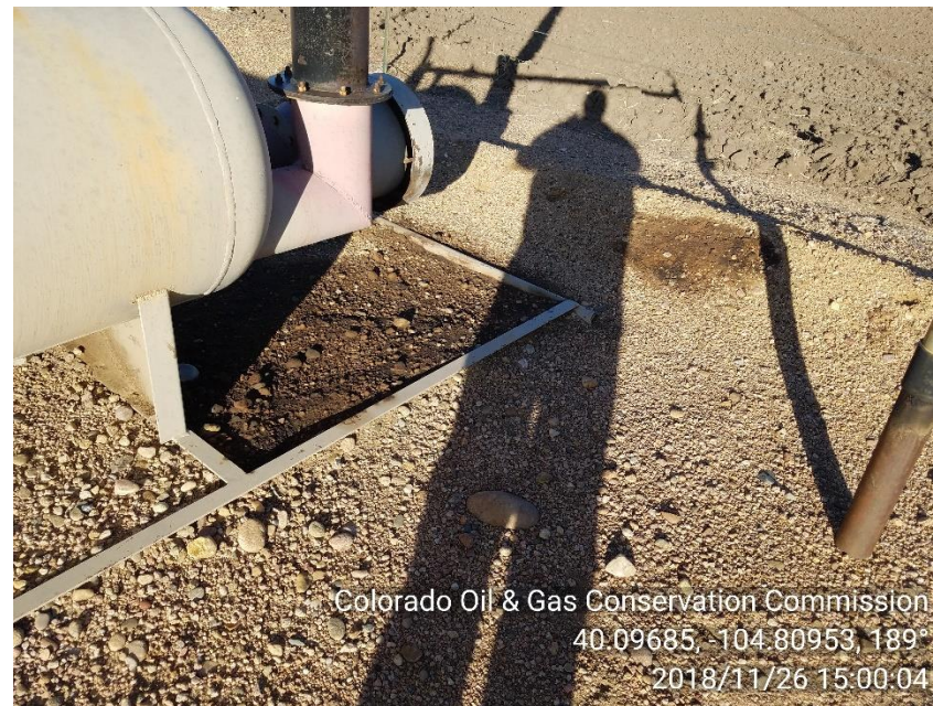
PHOTO 4: STAINED SOIL NEAR SEPARATOR
