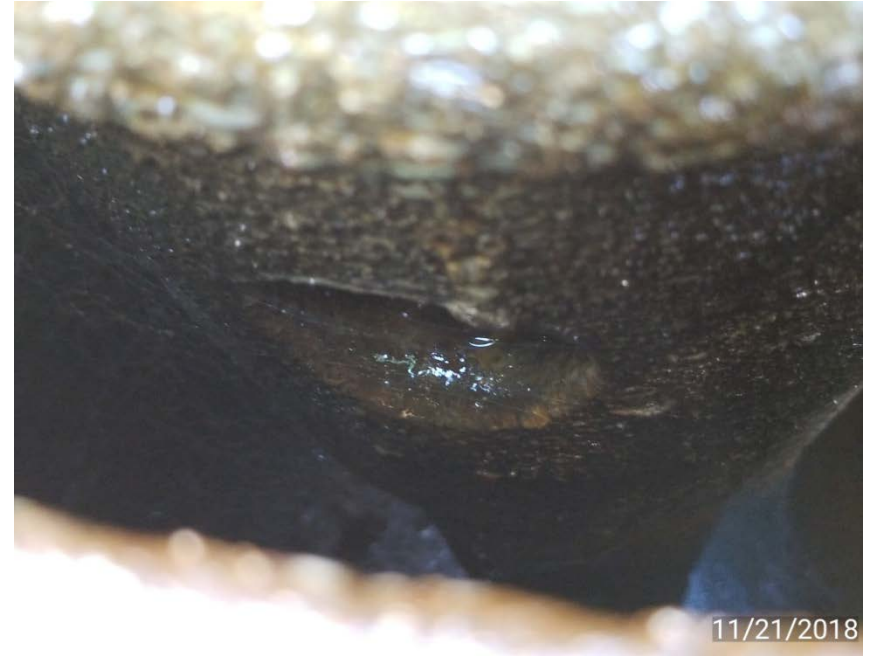
Photo 3. Casing open to atmosphere in cellar.
